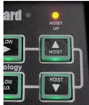
Hoist “Up” Indicator
